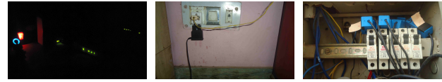
(a) Glowing LEDs in night (b) Wire snag leading to (c) Closely placed MCBs data loss causing interference
